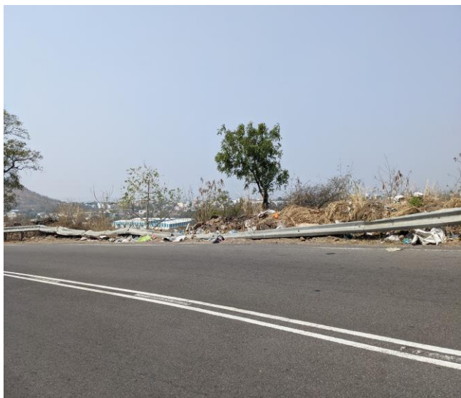
Image-3: Damaged and useless Side barrier
