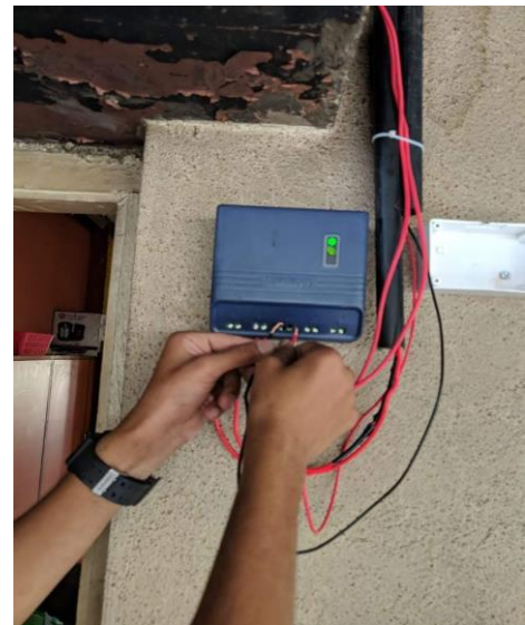
FIGURE 4:- INSTALLATION OF CHARGE CONTROLLER
